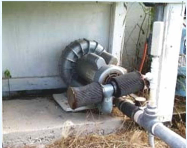
Figure 75: Air blower application in agitation plant
