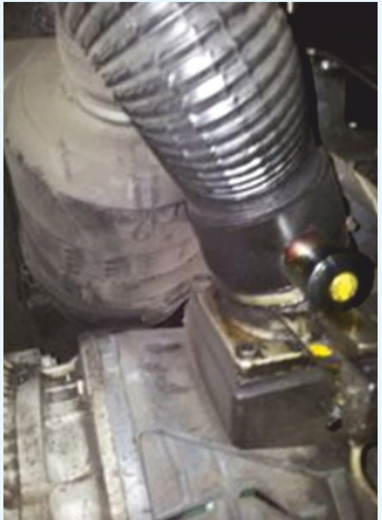
Figure 52: Screw Compressor Dusty and dirty
