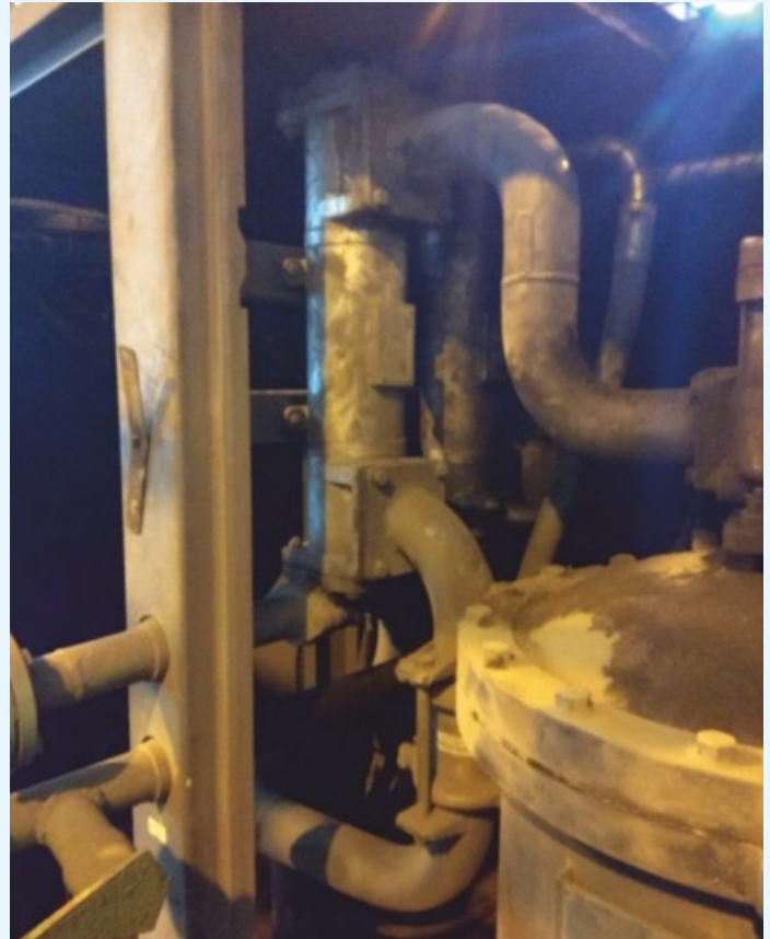
Figure 49: oil cooler, inter and after cooler
